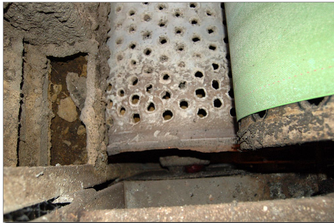
SMC WRC Belt Filter Presses (some units completely rebuilt 3 times)
