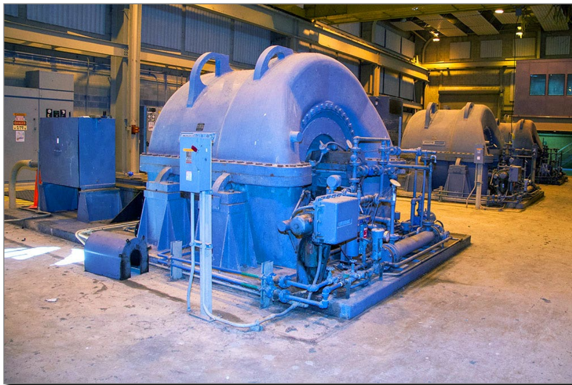
SMC WRC Aeration Blowers (original 1987 equipment)
